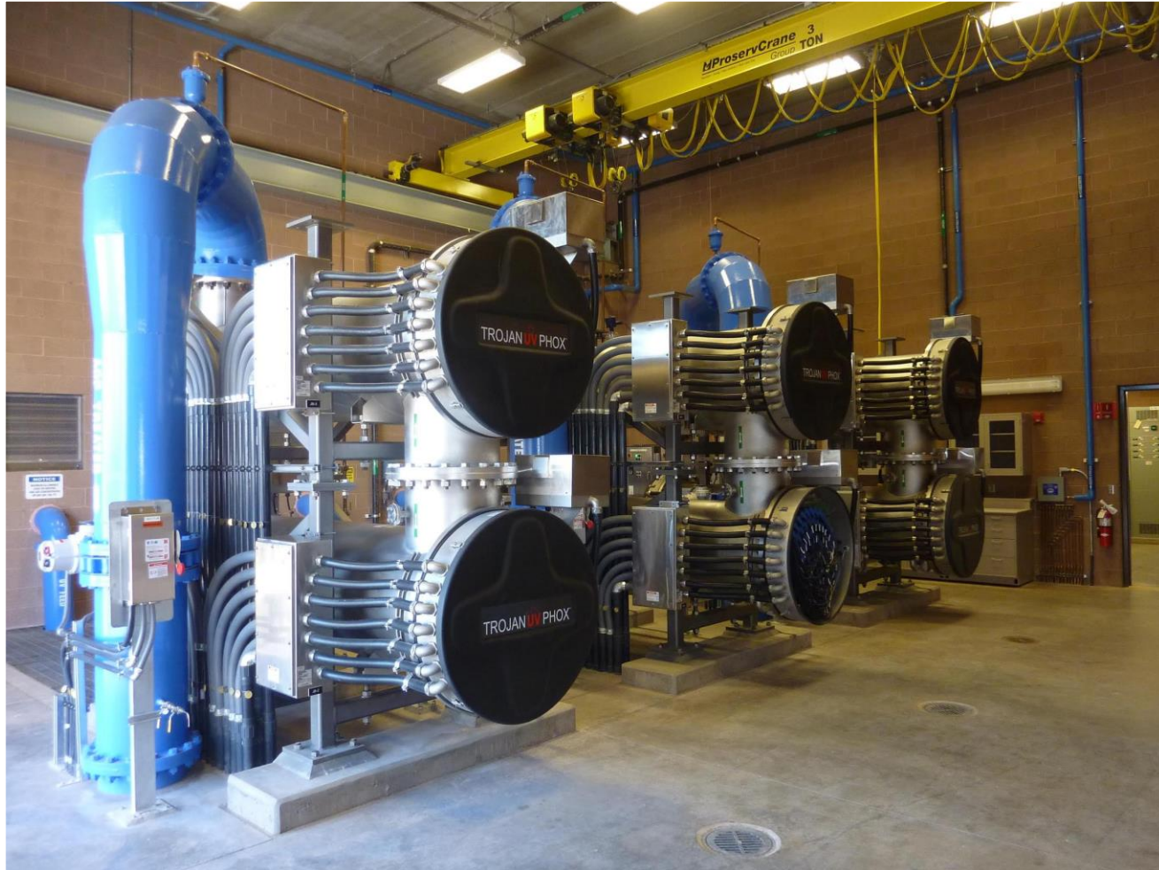
Advanced Oxidation Facility for Dioxane Treatment, Tucson, AZ
