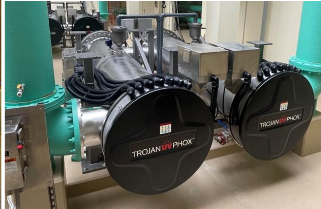
Advanced Oxidation Facility for Dioxane Treatment, Arden Hills, MN
