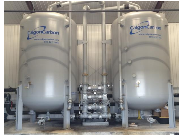
Full-scale GAC treatment of extracted groundwater
